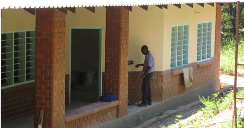
Electrician Liberty Muyamba working on the new Secondary Classroom Block at Limapela Cedric's
